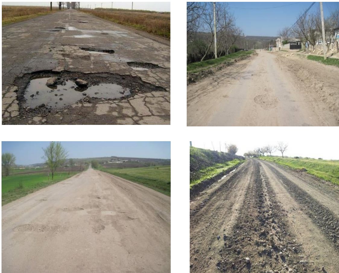
Figure 2-10: Damage to local roads
